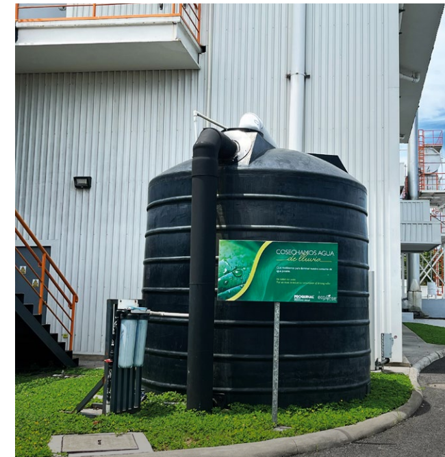
Rainwater collection tank | Costa Rica Plant
